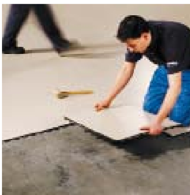
Laying when the business is still running: SILA K9 can be used immediately.
